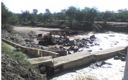
Figure 7: The destruction of the bridge due to flooding
